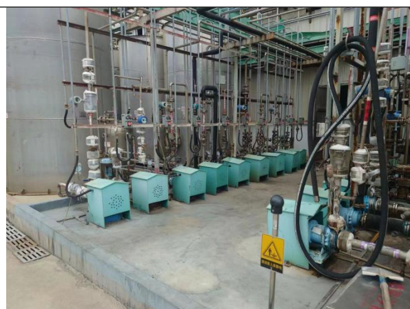
溶剂回收车间传输泵
