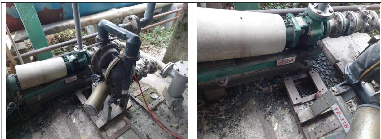
污泥浓缩池传输泵
